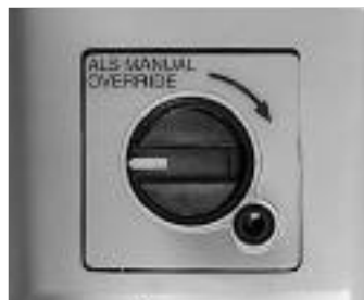
Convert from BLS to ACS operation with a turn of this switch.
